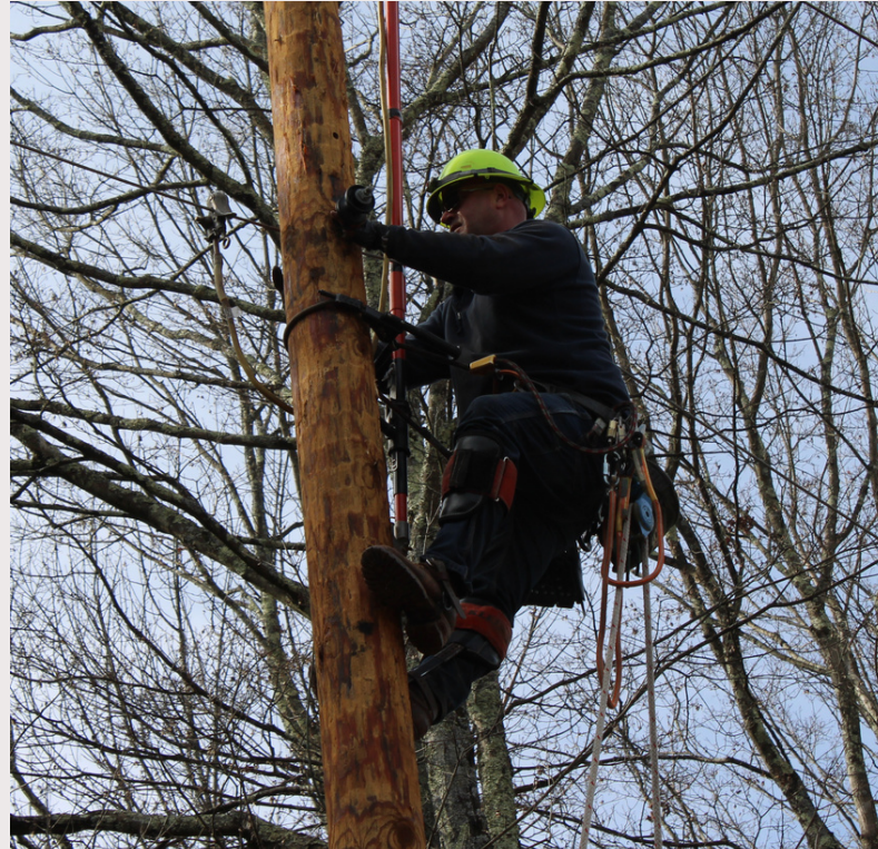
Above: Senior lineman Chad Phillips finishes up a new service pole for a seasonal residence.
