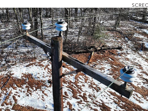
BIRD'S-EYE VIEW: This image, captured by Zeitview drones in 2024, shows a broken conductor tie wire (right insulator), which holds the electric line to the insulator, and two areas of decay on the crossarm. From a ground inspection, the decay would not have been visible.
