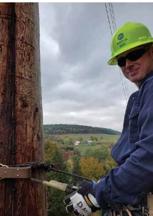
POLE PATCHES: During the time a substation is off-line, co-op lineworkers, including Dave Kepner, make needed repairs such as patching holes on poles caused by woodpeckers.
